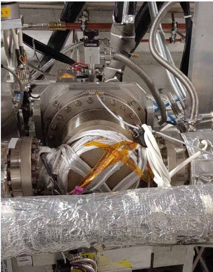
A PPS Roman pot containing a diamond-based time-of-flight detector module in the LHC tunnel for the 2023 high luminosity running.
